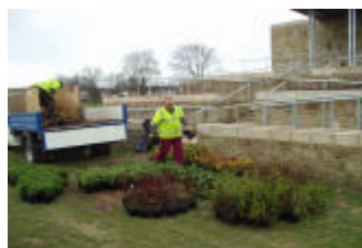
Planting of terrace at new changing rooms, King George V Playing Field
